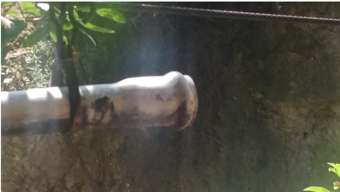
The House Tunnel supply line pulled apart and a bell and spigot joint
