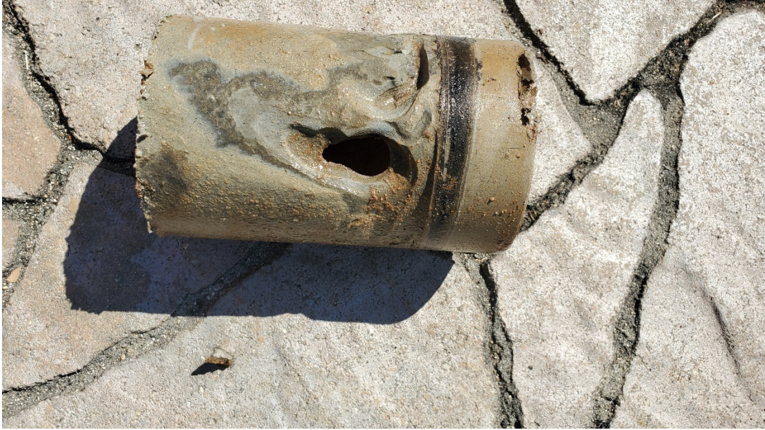
Cause of water main leak on Mesaloo Lane
