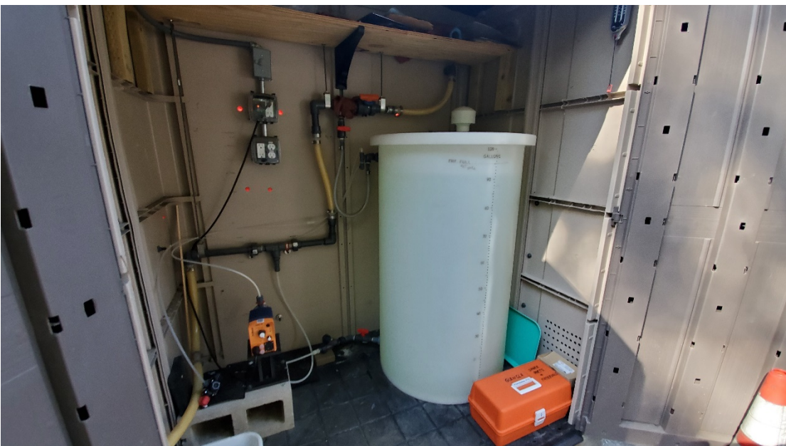
Chlorine Storage Tank
