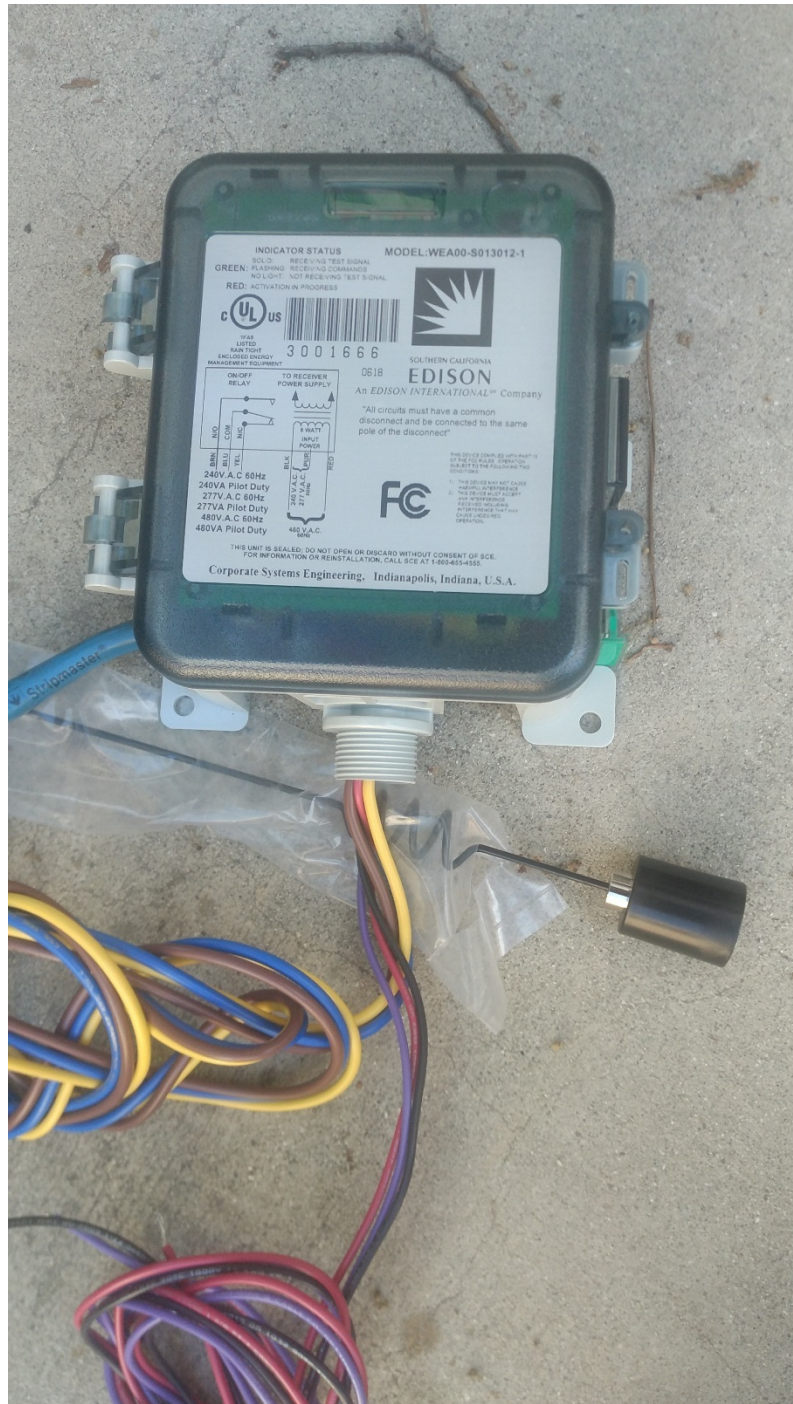
Installation of new radios at three sites for the agriculture and pumping interruption (API) rate reduction program
