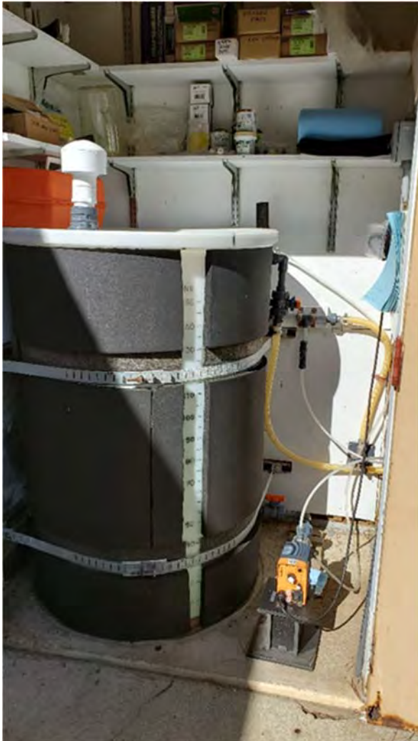
Chlorinator building with storage tank and metering pump
