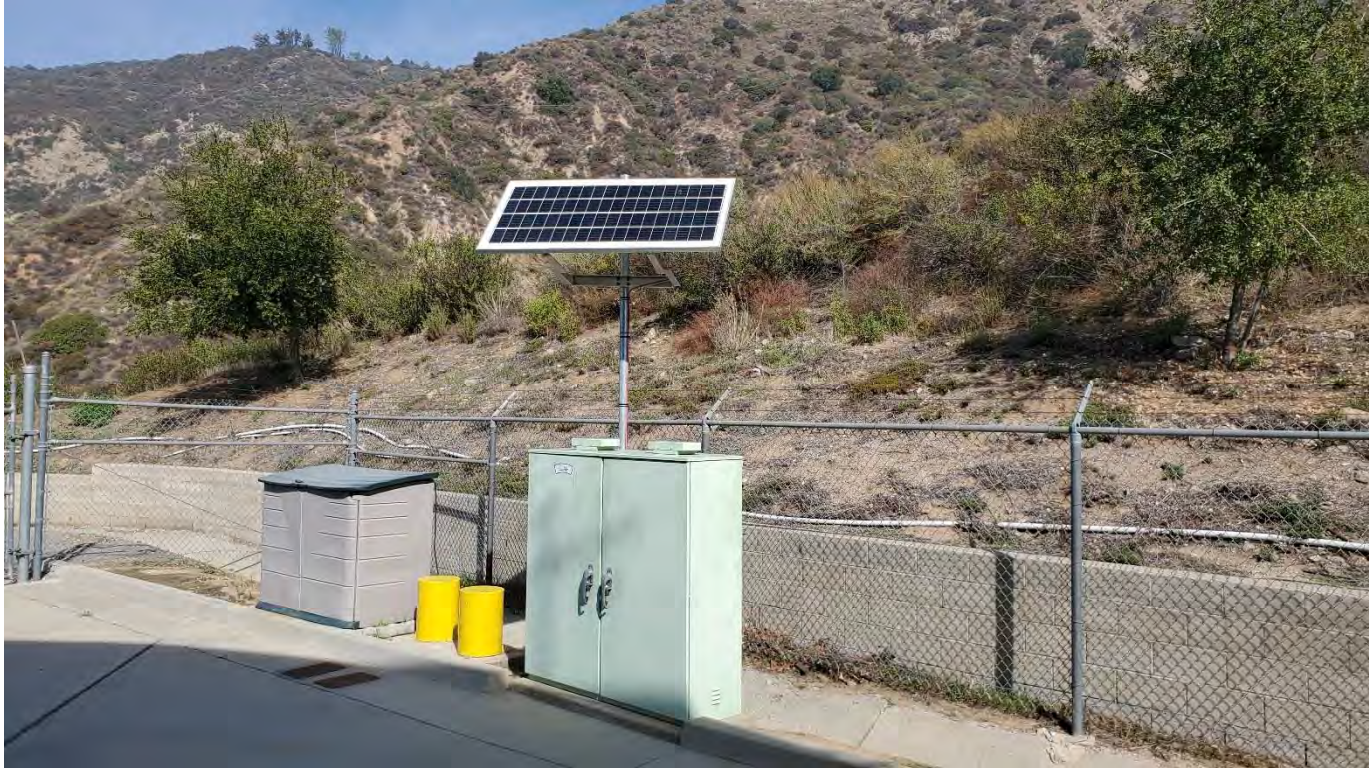
Solar Power Supply installed at West Tank
