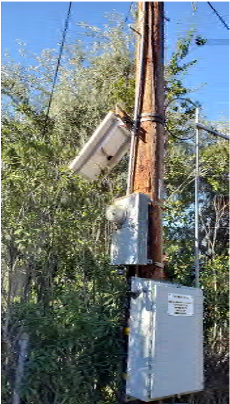
Solar Power Supply installed at Transfer Valve
