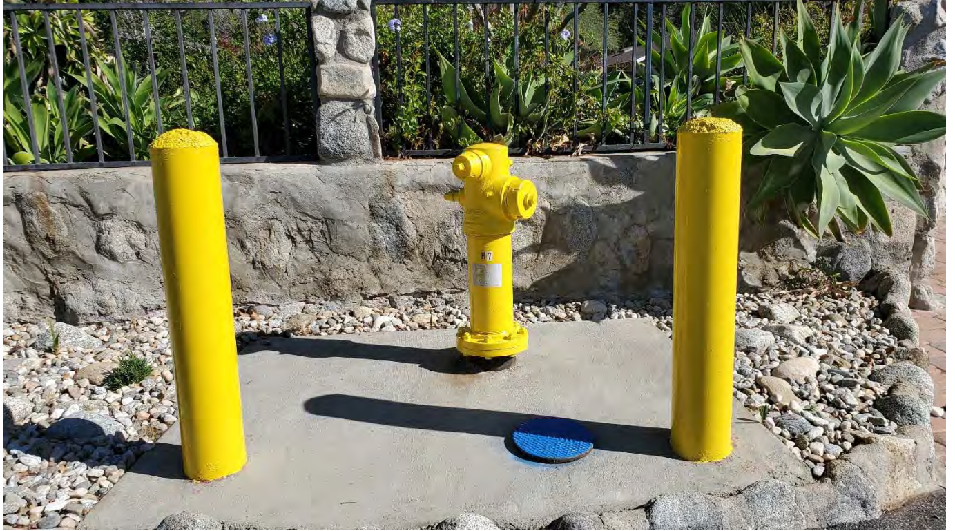
Fire Hydrant maintenance program which includes labelling, painting and testing
