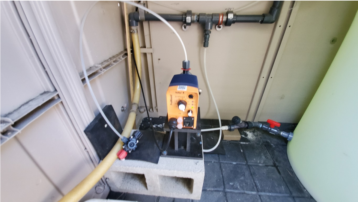
Chlorine Metering Pump
