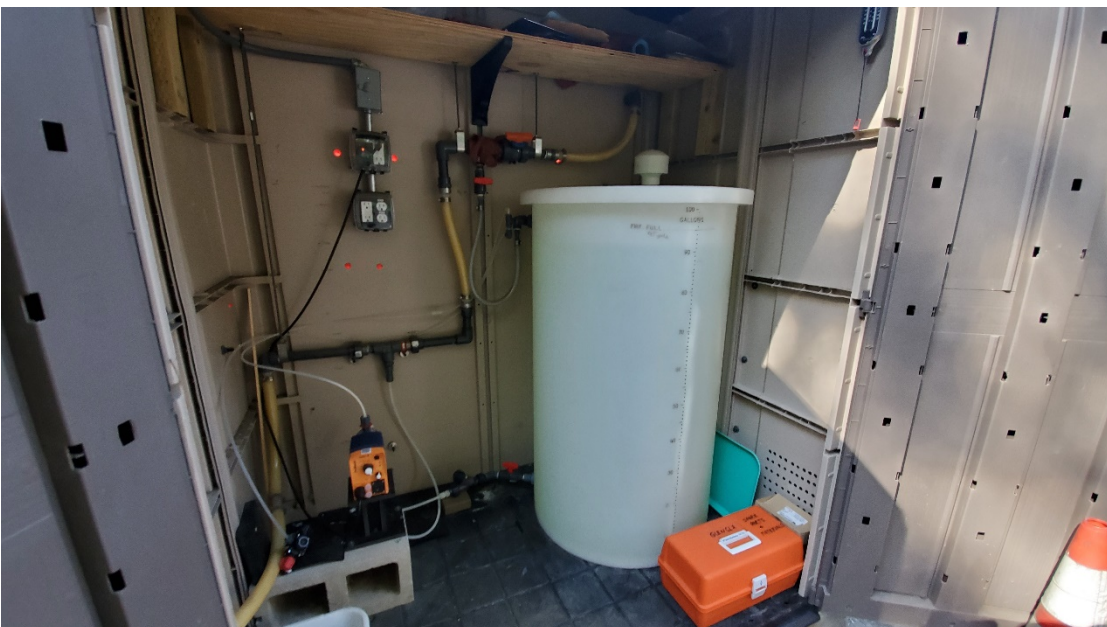
Chlorine Storage Tank
