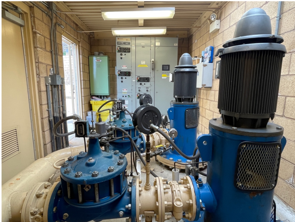
Figure 2-17. Sage Booster Pump Station View 2
