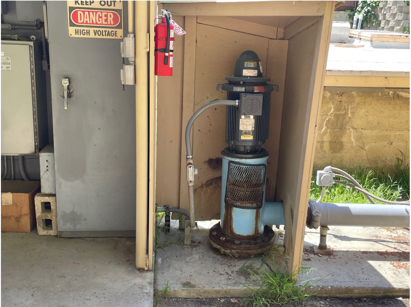
Figure 2-20. Glen Booster Pump Station
