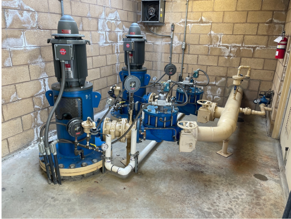
Figure 2-16. Sage Booster Pump Station View 1
