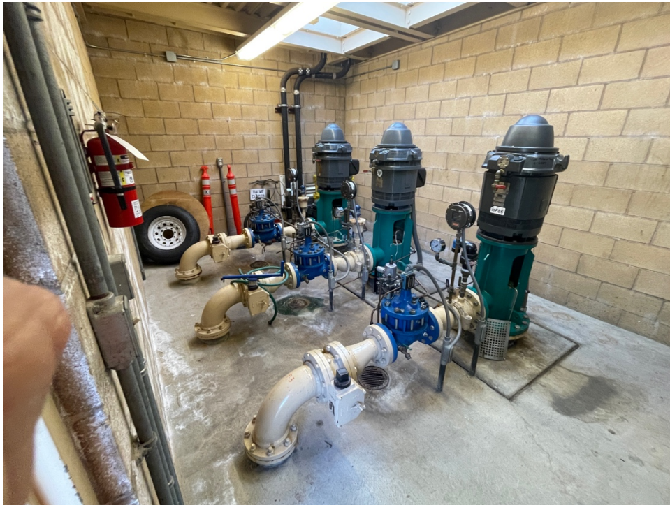
Figure 2-15. Eucalyptus Booster Pump Station View 2
