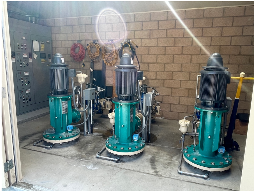
Figure 2-22. Vosburg Booster Pump Station View 2
