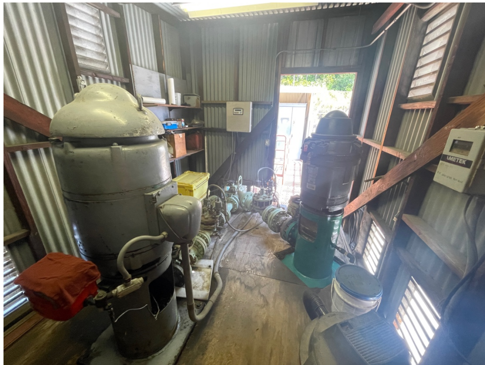
Figure 2-19. Wilcox Booster Pump Station View 2
