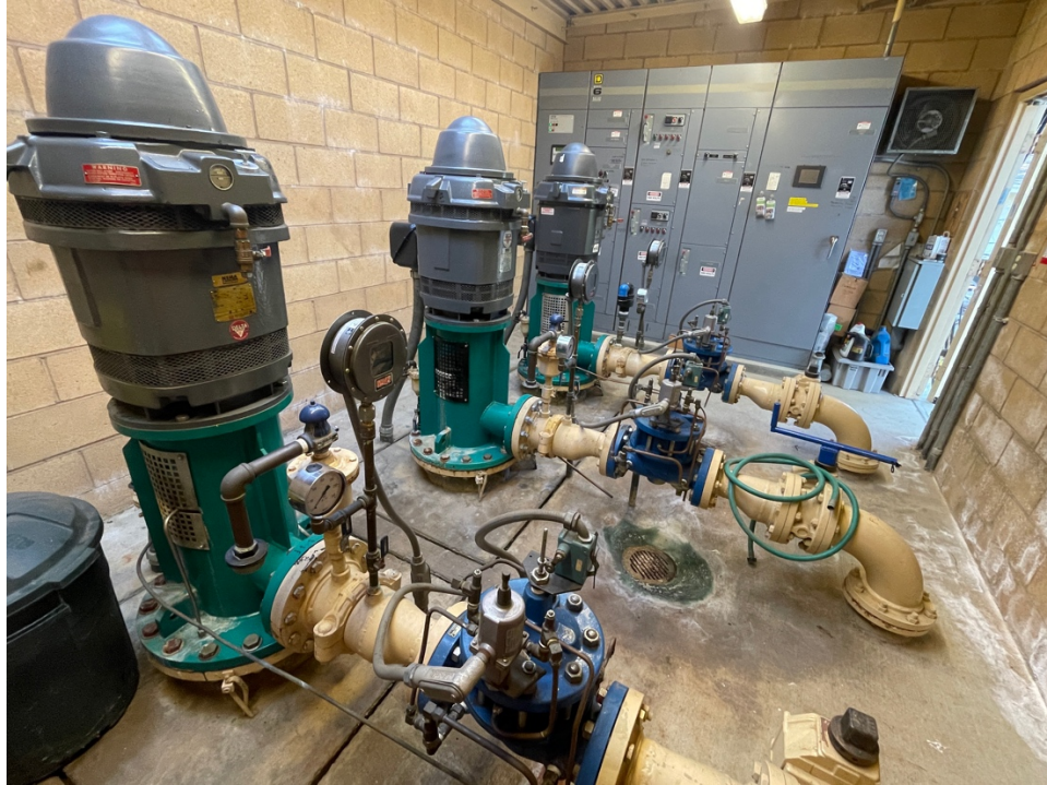
Figure 2-14. Eucalyptus Booster Pump Station View 1
