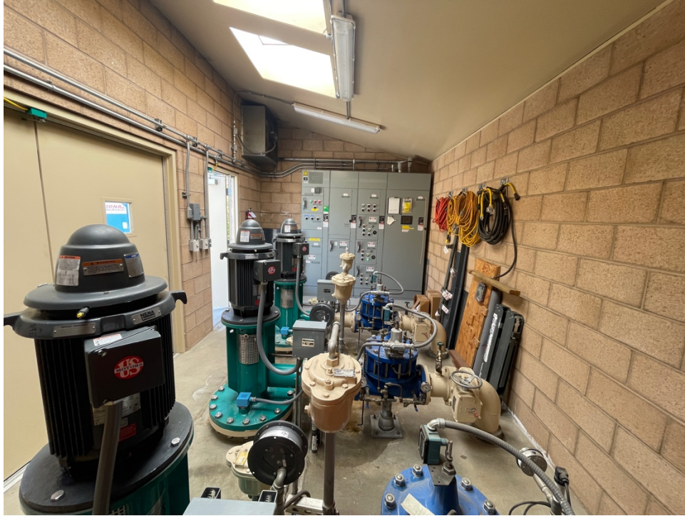
Figure 2-21. Vosburg Booster Pump Station View 1
