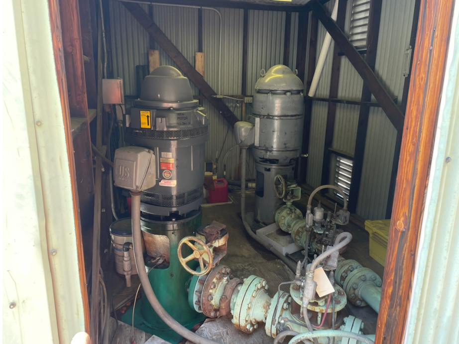
Figure 2-18. Wilcox Booster Pump Station View 1
