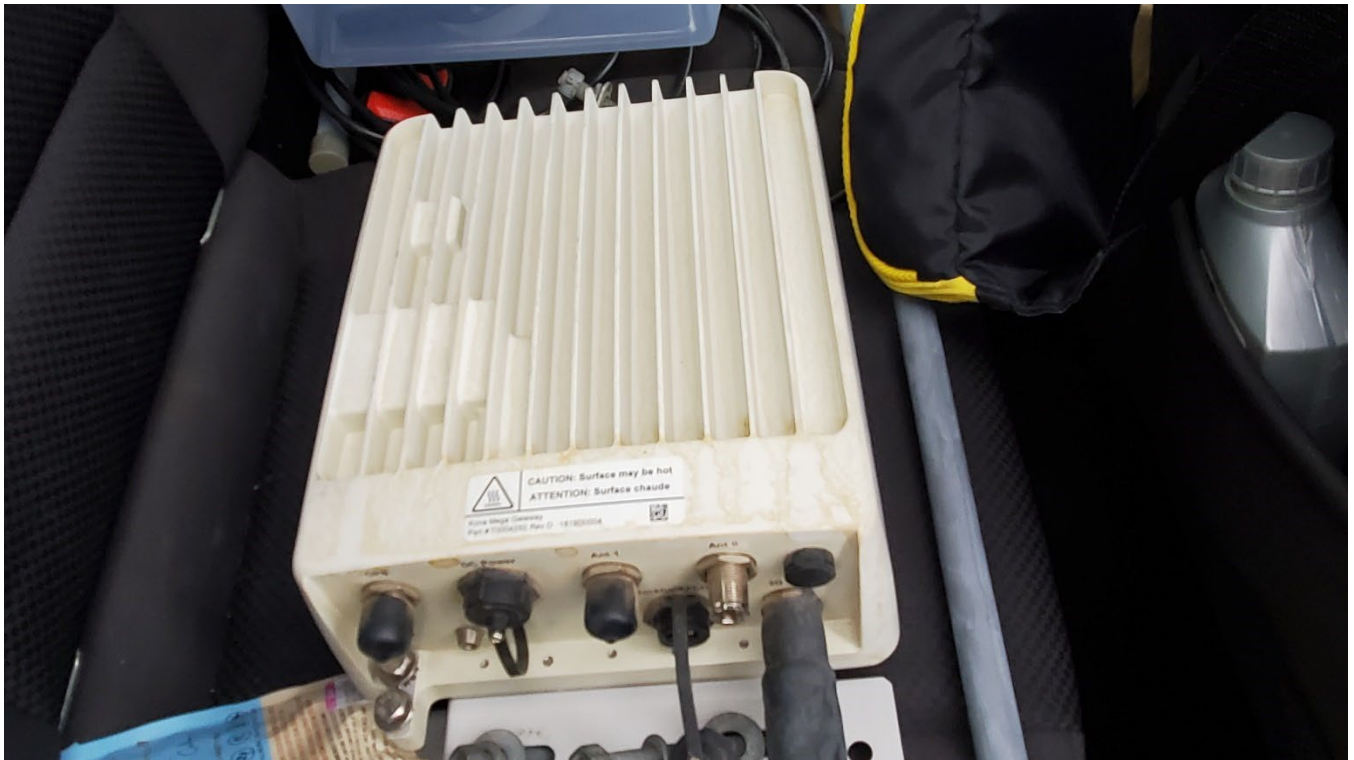
The District's communication gateways use the LoRaWAN ® specification, which is a Low Power, Wide Area (LPWA) networking protocol designed to wirelessly connect battery operated 'things' such as our AMI devices to the internet and provide bi-directional communication, and end-to-end security.
