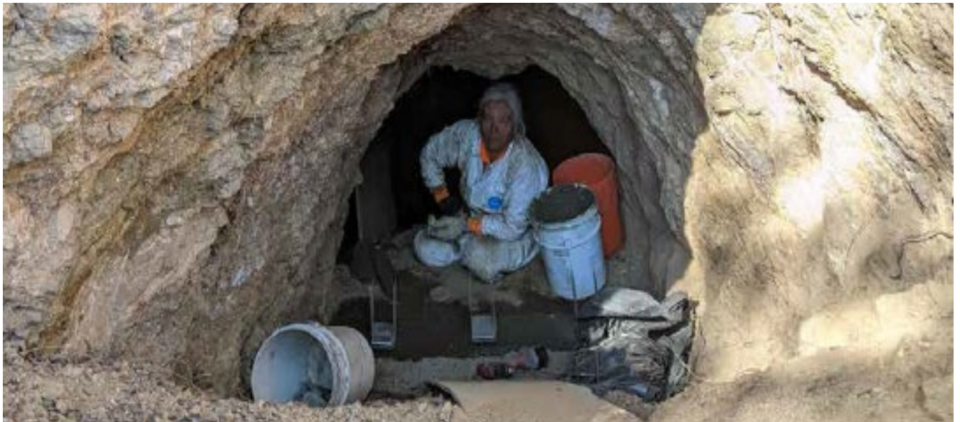
House Tunnel and its pipeline were restored to provide a supplemental water supply.
